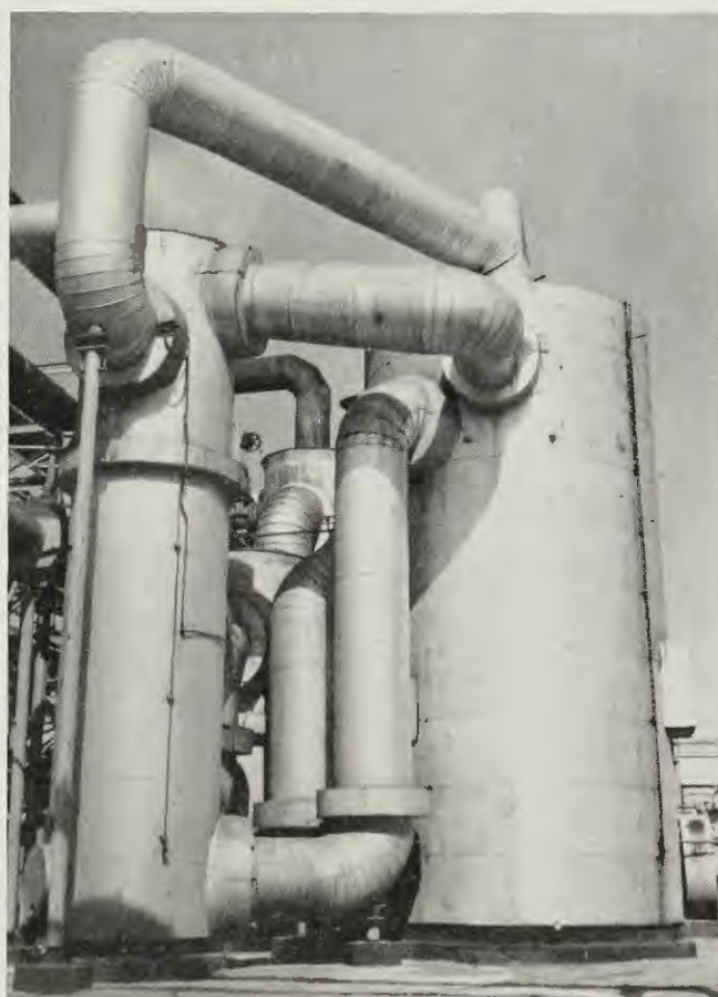
Hot heat exchanger (left) and converter in the Acid plant.
