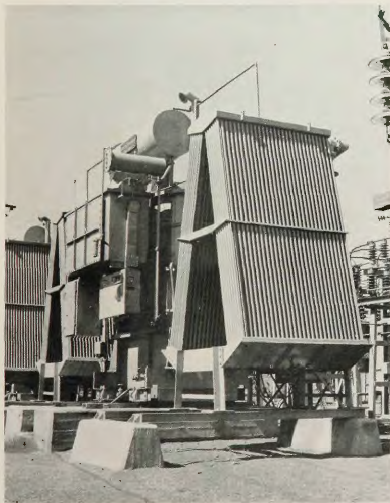
Transformers, such as these at Broadmeadow, supply power for many of Newcastle's great industries.
