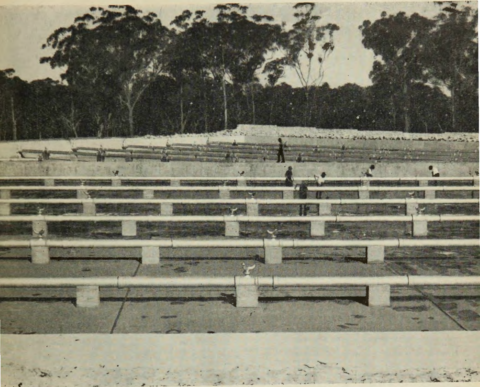
Aeration Pipes at the Tomago Sandbeds.
